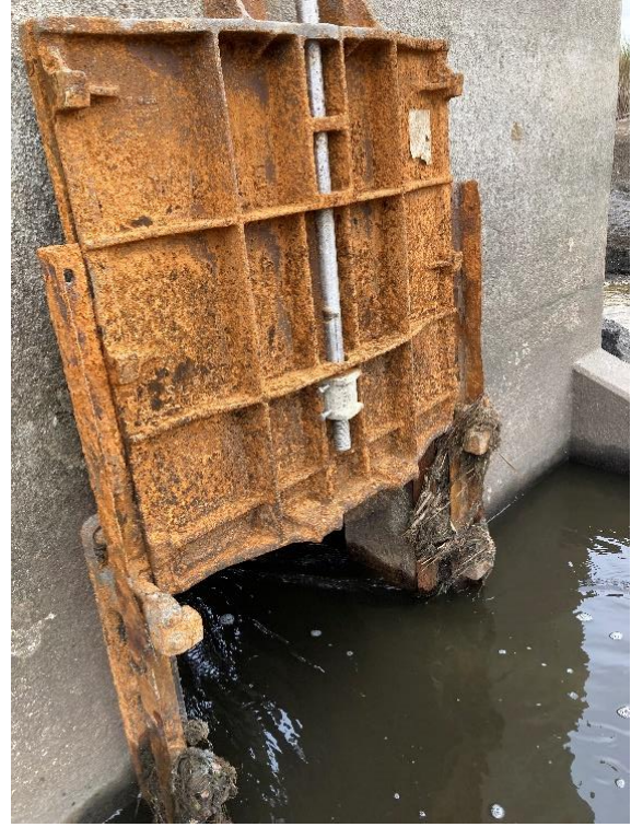
Figure 10 – Sluice Gate Front
